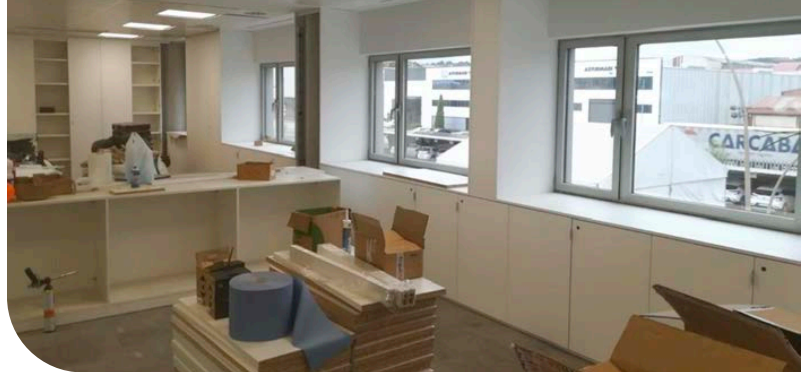
Remodelación interior de la sede de la APA. Inner remodelling work of the Port Authority's headquarters.
